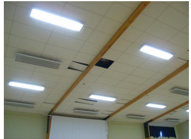
(d) No damage to portal frames despite ceiling tiles displaced by shaking.
