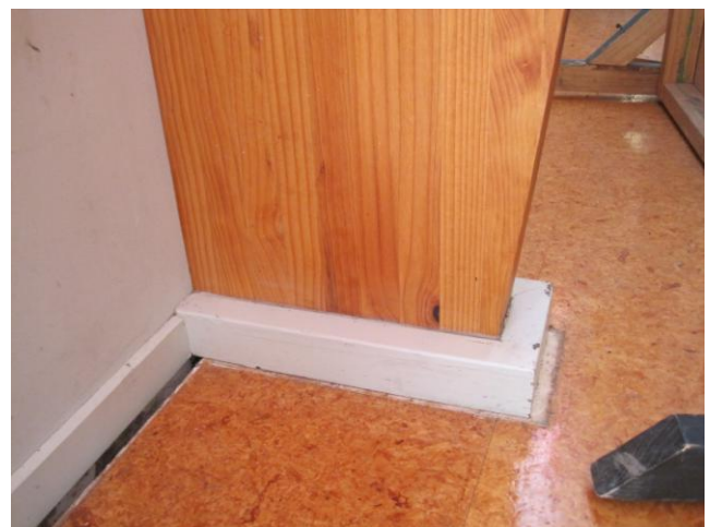
(b) Minor lateral movement of foundations.
