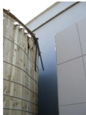
Figure 12: Damage to 210 m 3 , 7.75 m diameter tank in Hornby caused by a 3 sec slosh wave in the 2010 earthquake. The liner ruptured. The broken timbers have been replaced and the tank is working again now with a baffle system installed.
