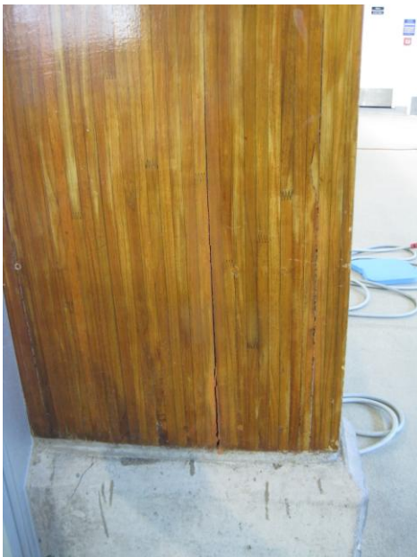
(a) Re-opening of old shrinkage crack at epoxy rod connection to foundation.
