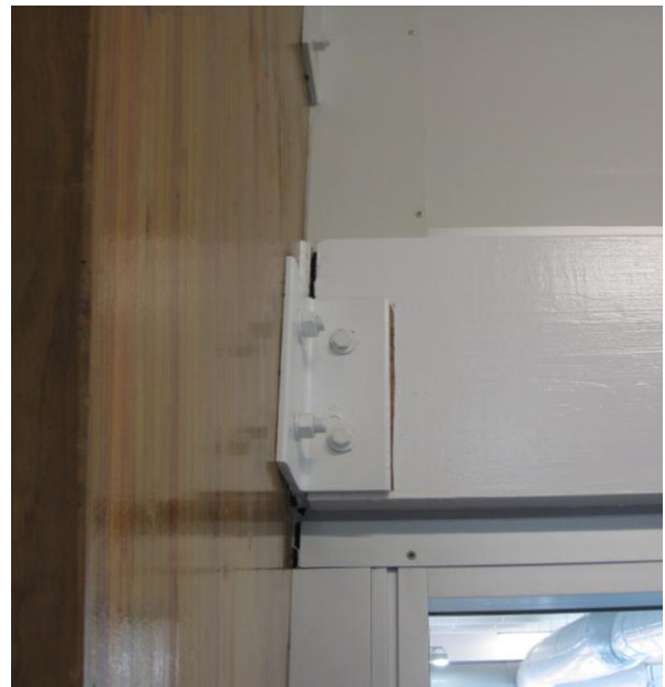
(b) Minor gap opening due to lateral movement.
