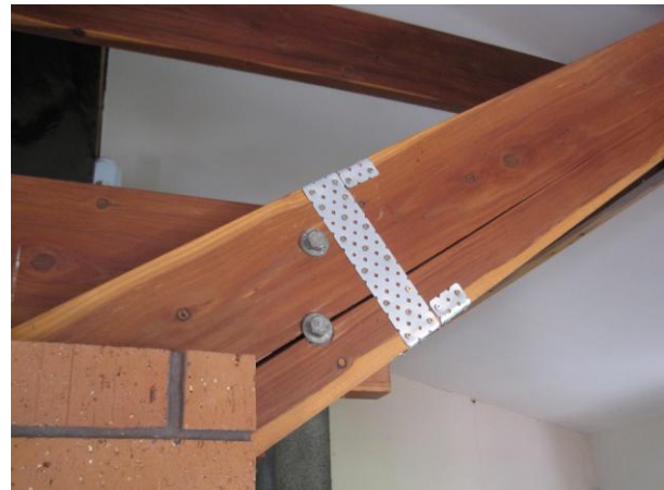
Figure 8: Emergency repair to a bolted rafter connection in a private house.
