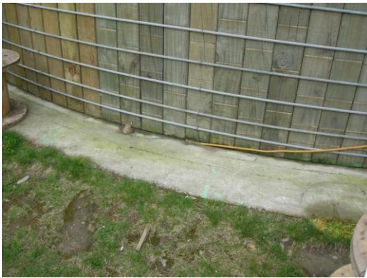
(a) Base Isolation sliding of 50 mm for 400 m 3 tank in Kaiapoi. No damage to tank.
