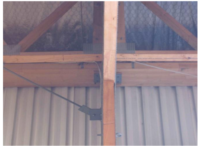
(b) Local lateral displacement of rafter at knee joint.
