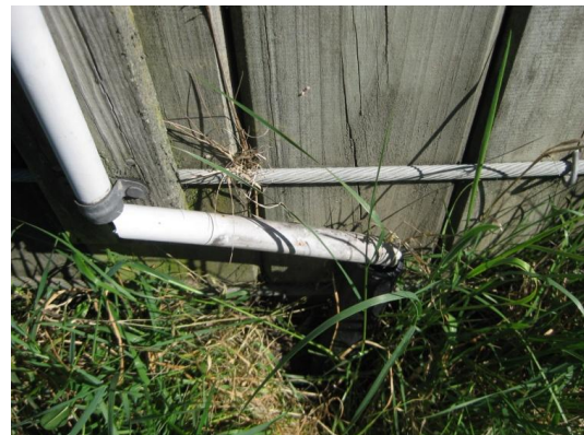
Figure 11: Pipe damage due to rotation of 100 m 3 tank at West Melton. No damage to tank.
