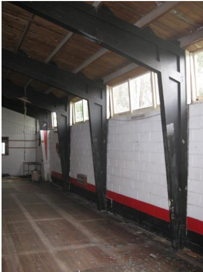
(a) Timber frames with damaged masonry infill walls.
