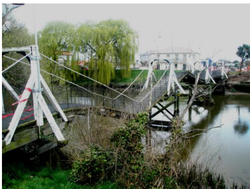
(a) Damage to Mandeville Bridge following 2010 earthquake.
