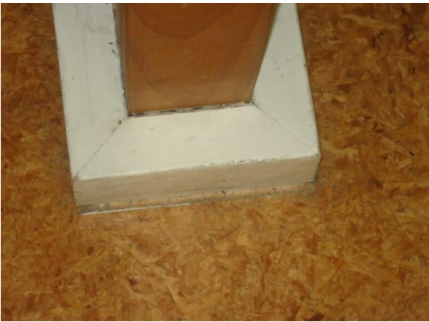
(c) Minor foundation movement visible at floor level.
