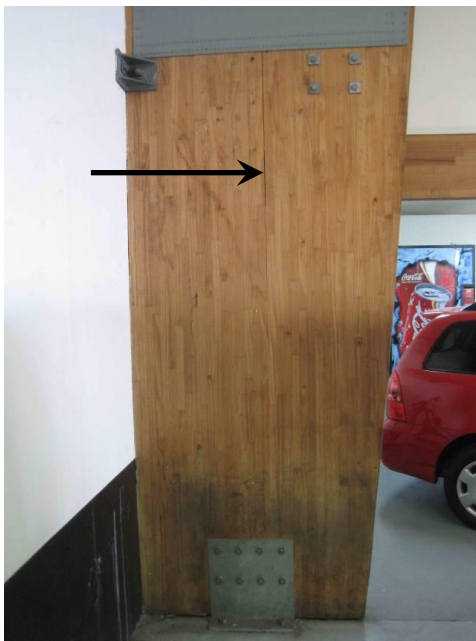
(c) Vertical shear crack in column (location shown by arrow).
