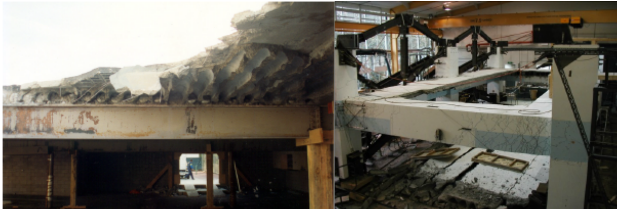
Figure 2: Photographs of damage to precast concrete floor systems. Left shows the Meadows Apartment Building, California, as a result of the 1994 Northridge earthquake. Right shows Matthews super-assembly specimen at the completion of the Phase 1 testing. Note the specimen’s floor dropped out at a low seismic load with little damage to the surrounding frames.
