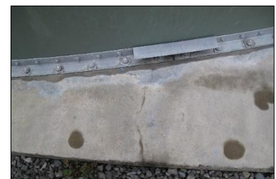
(c) Minor cracks on concrete slab
