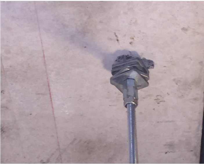
Figure 11: Poor installation. If in doubt, chuck in more washers
