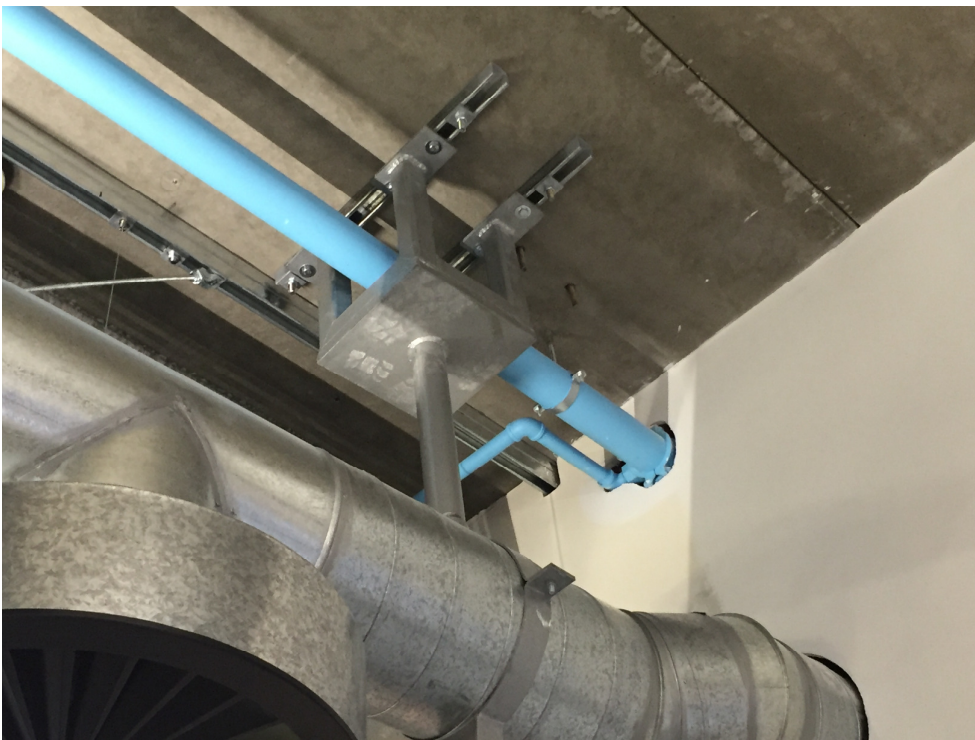
Figure 7: Specific solution for area where services clashed and could not be moved
