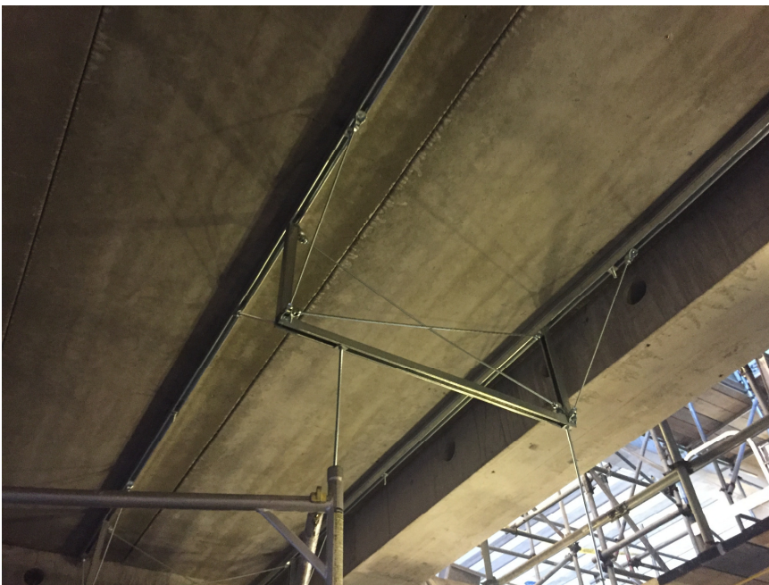
Figure 8: Simple configuration on unistrut lengths off underside of slab, to allow for some positional tolerance
