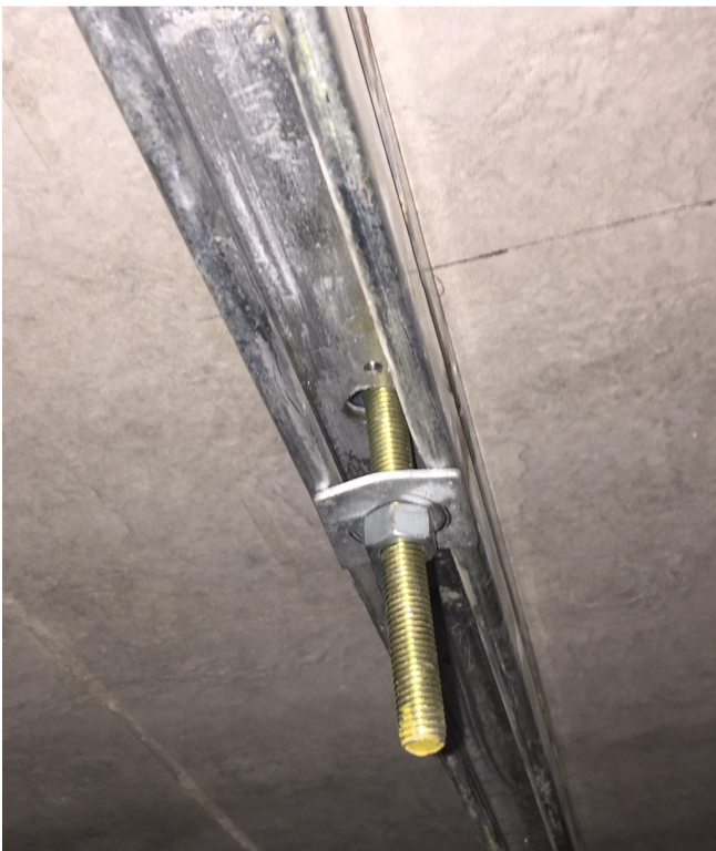
Figure 9: Wrong sized washer that got bent during installation
