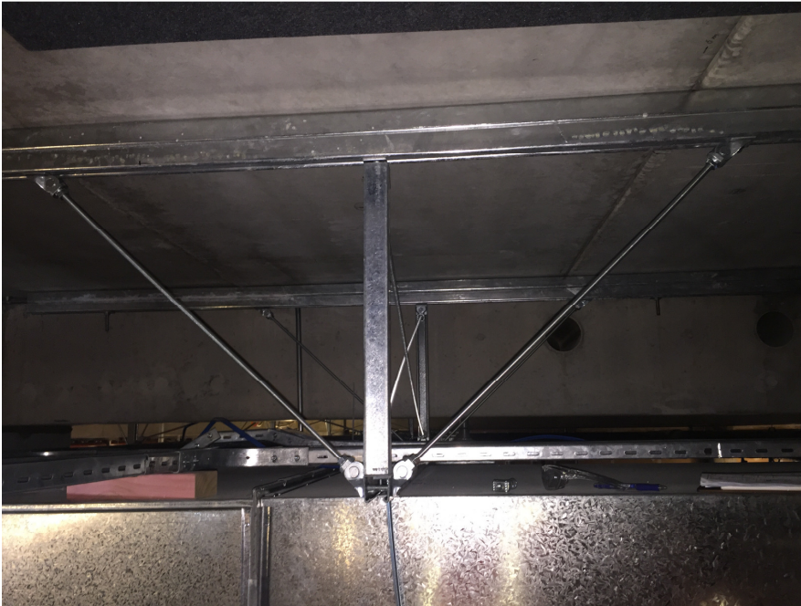
Figure 4: Simple configuration on unistrut lengths off underside of slab, to allow for some positional tolerance
