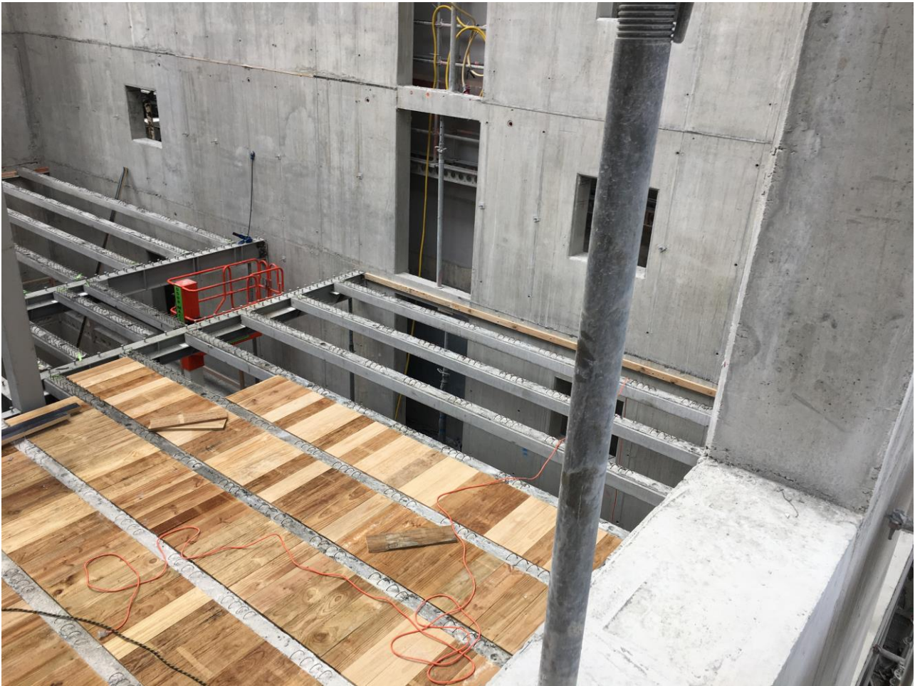
Figure 6: Rib-Infill floor prior to installation of topping diaphragm. The floors were installed following construction of the exterior walls and connected via cast-in Ancon threaded couplers.
