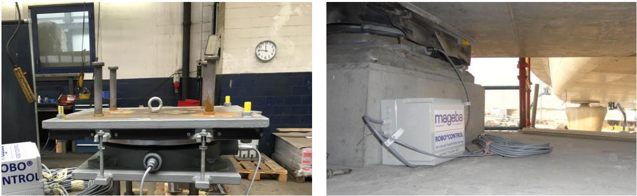
Figure 3: Testing of the load-measuring functionality and performance of a spherical bearing (left), and one of the SHM system's 14 control boxes and its connection to the spherical bearing above it (with dust skirt)
