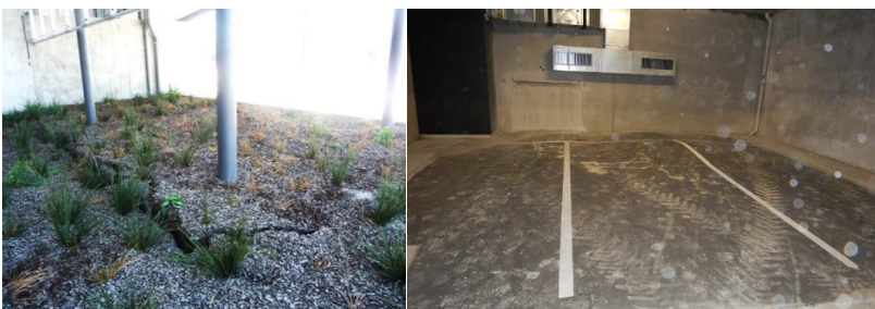
Figure 4: Ground surface disruption (left); pavement bulging between ground beams (right)
