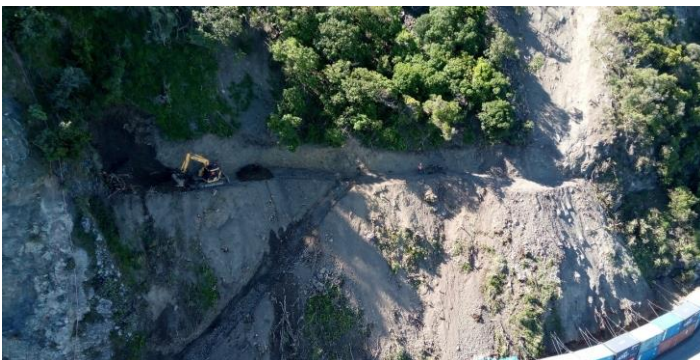
Figure 4: The bench and access ramp enable for improved access for the fence installation
