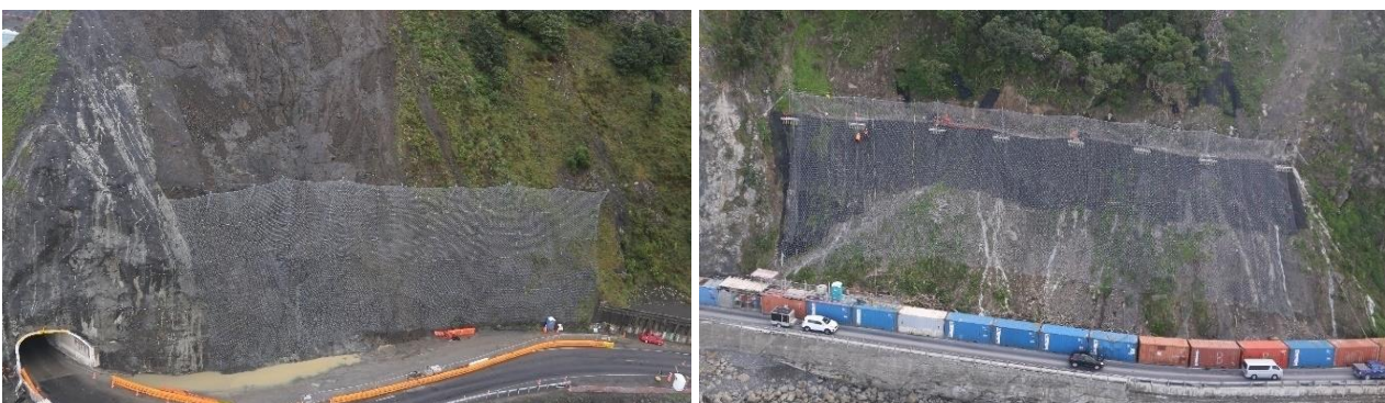
Figure 5: (Left) SR14, installed across a planar slope (Right) SR18/19, constrained by complex topography
