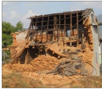
(b) Out-of-plane collapse of wall led to collapse of roof and floor, 2015 Gorkha earthquake, Nepal
