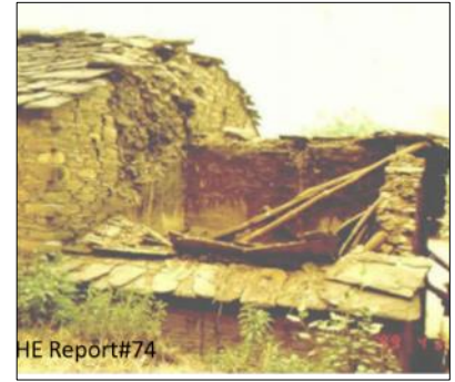
(f) Roof collapse due to absence of wall-roof connections, 1999 Chamoli earthquake, India (Photo credit: WHE, Report # 74)
