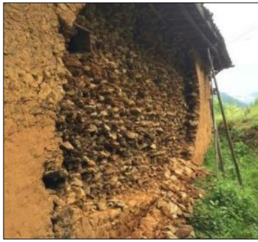
(a) Delamination and bulging of wall wythe, 2015 Gorkha earthquake, Nepal
