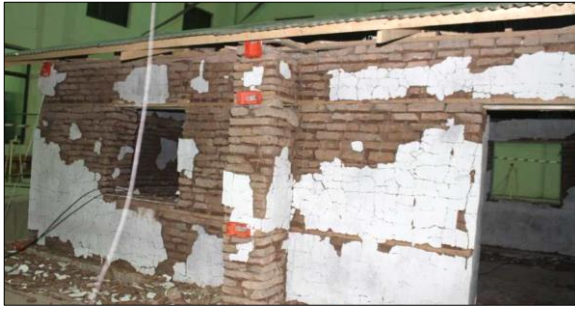
(e) Out-of-plane movement face-loaded wall (DT 4)
