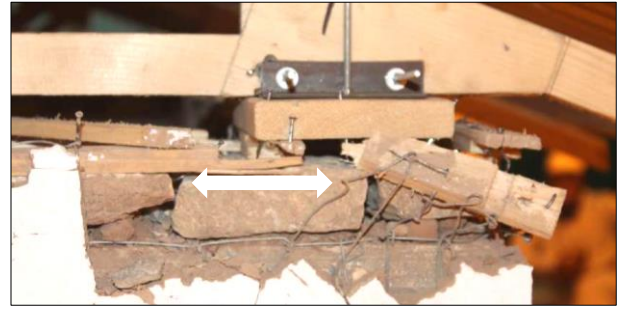
(f) Breaking of timber band (DT 4)
