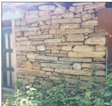
(a) Intermixing of double and single thickness stones
