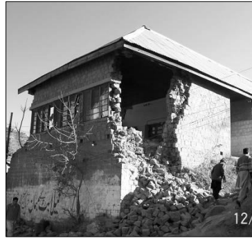
(e) In-plane wall and corner damage, 2005 Kashmir earthquake, Pakistan
