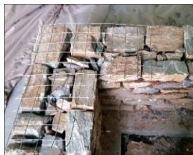
(b) Close-up view of stone wall (wire mesh on the wall is stitch) (DT 2)
