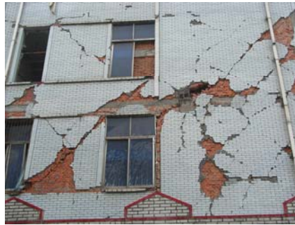
Figure 1: Damage of RC building with masonry infill walls in China 2008 Wenchuan Earthquake
