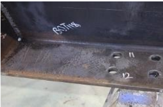
Figure 19: Damage in flange in smaller member
