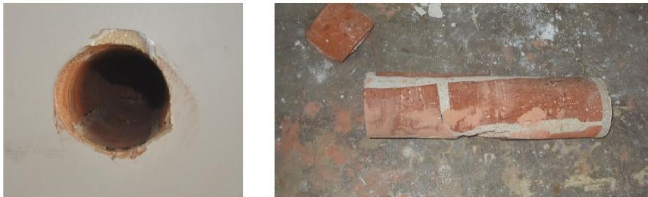
Figure 6: Photos of existing URM interior wall core samples, illustrating their solid construction with no internal cavity.
