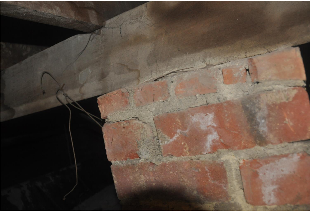
Figure 7: Photo of existing timber bearer on URM supporting pier. No tie or direct fixing is evident.
