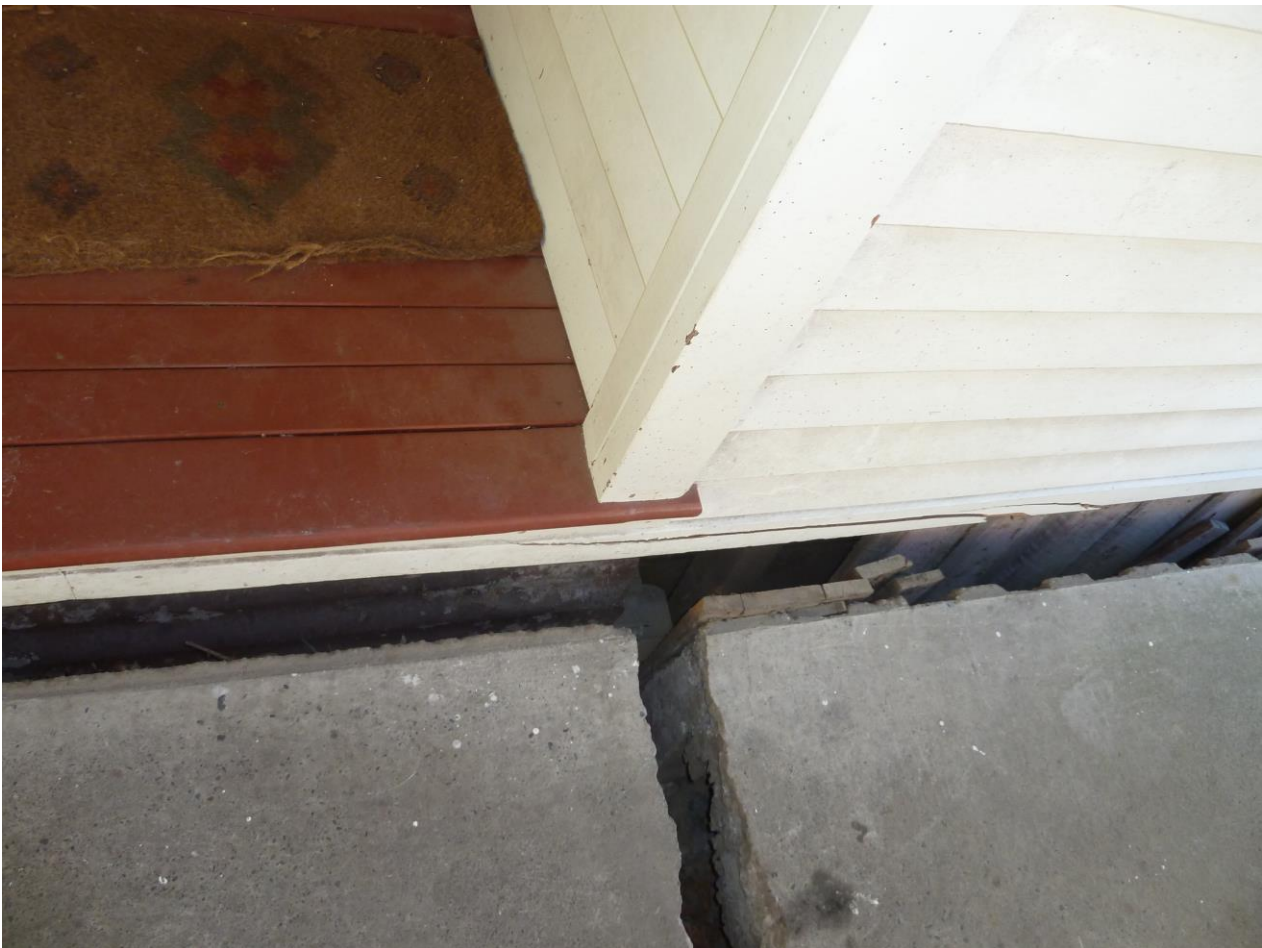
Figure 2: Downslope displacement of footing on uphill side
