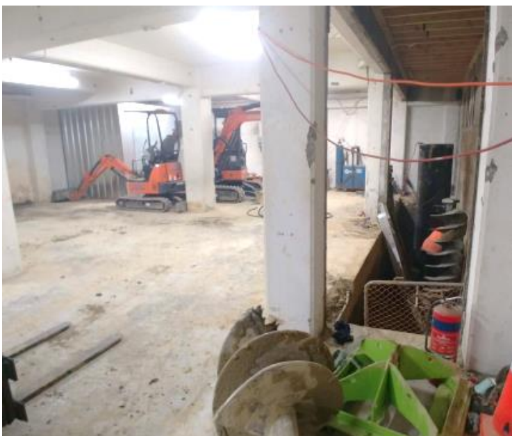
Photograph no. 3: Enabling works to increase working head room via trenching into the ground and removing ceiling panels. Trenching works also exposed existing foundation pads for examination
