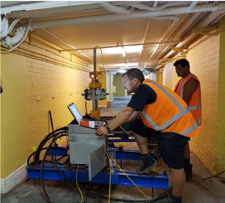
Photograph no. 1: A portable CPT rig (1.2m wide, 1.6m long) operating within a 2m wide basement tunnel with a limited head room of 2.5m
