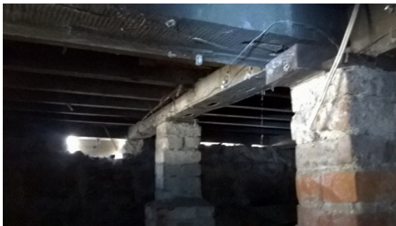
Figure 15: Foundation system – bearers and wall bottom plates all of different sizes (note the packing off the piles), supported on URM piles.
