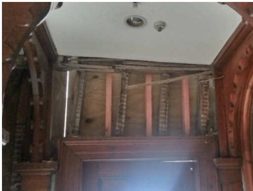
Figure 9: Jack studs in timber walls displaced
