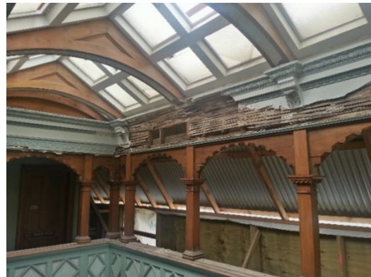
Figure 10: damage to lathe and plaster linings in atrium
