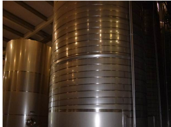
(b) Buckling of tank wall
