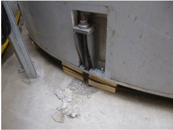
(a) Combined concrete cone-pull-out failure
