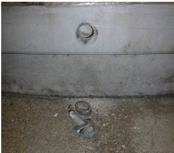
(c) Steel shear bolt failure
