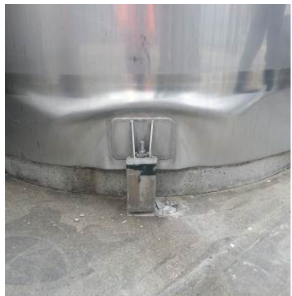
(f) Local buckling of skirt
