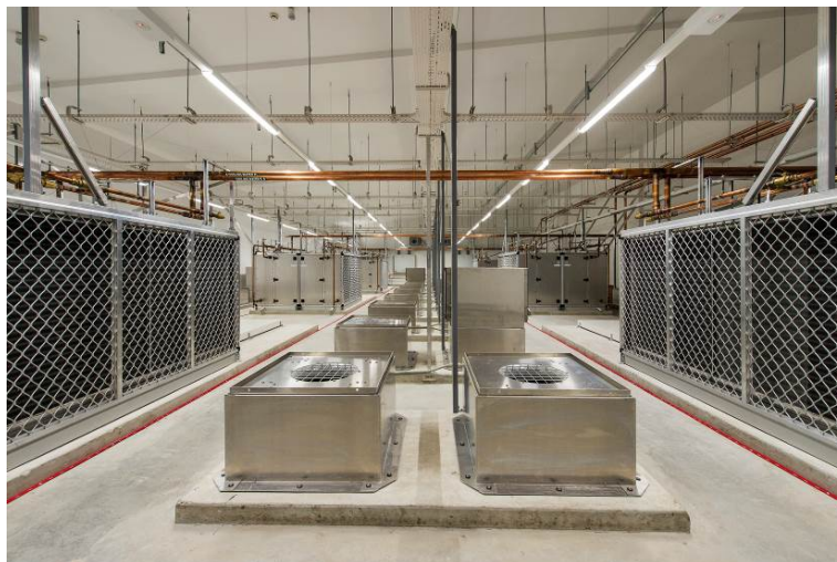
Figure 2. Interior view of plant room. Floor accelerations significantly reduced the need for lateral bracing of building services.
