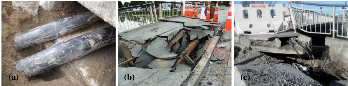
Figure 1. Utility failures at bridge crossings, after the CES; a) Partial failure of 66KV lines at Dallington Bridge (Eidinger and Tang, 2012); b) Damage to pipelines crossing over Avon River (Cubrinovski et al. 2011); c) Damage to lifelines at Gayhurst Road Bridge (Palermo et al. 2012).
