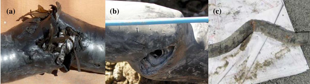
Figure 5. Damages to cables during the CES; a) Failure of 66 kV oil filled cable (Eidinger 2012); b) Failure of 66 kV XLPE cable (Eidinger2012); c) Failure of 11 kV cable (Eidinger and Tang 2012).
