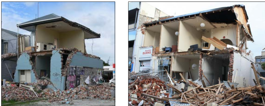
Figure 1. Observations of URM building damage with non-loadbearing partition walls from 2011 Christchurch earthquake.
