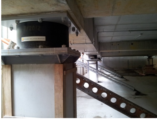
Wynn Williams House, Christchurch, Alteration of the treatment of the displacement window through base isolation.
