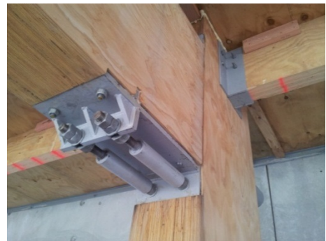
(c) Detail of exposed yielding devices with epoxied connection into the post-tensioned beam.
