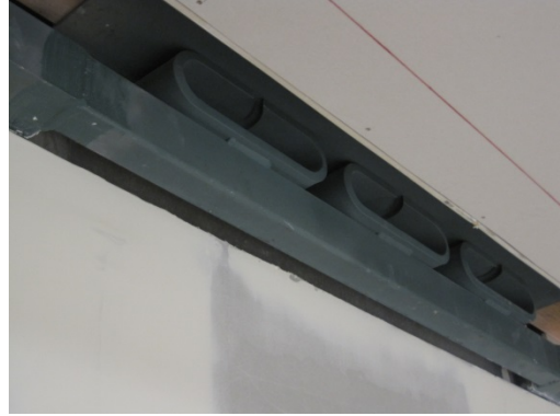
CoCA building, Massey University, Wellington, Concentration of dissipative devices at first floor level.
