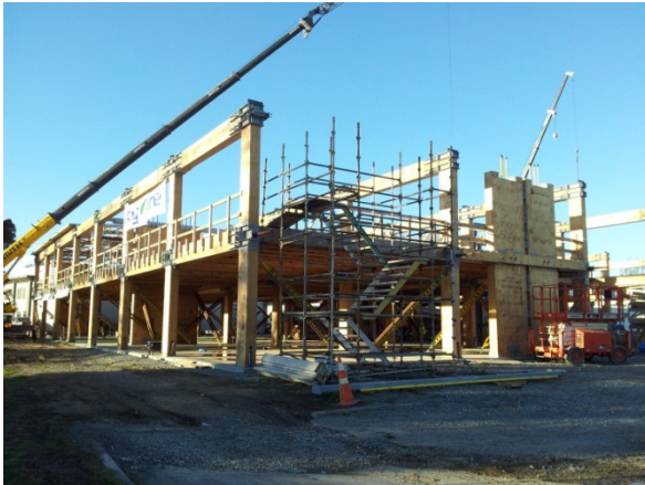
Office building for Trimble Navigation, Christchurch, increased stiffness of the columns by specifying stiffer timber material.
