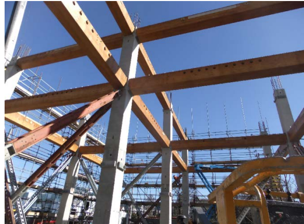
Wynn Williams House, Christchurch, increased stiffness of the columns by specifying reinforced concrete.
