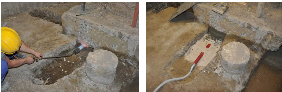
Figure 4. Scorching of the base and installing of a pressure cells below an existing spread footing (MF1).
