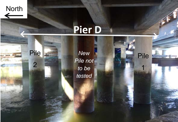
Figure 2. Elevation of Pier D as viewed from Abutment F (Photo taken 20th May 2014).
