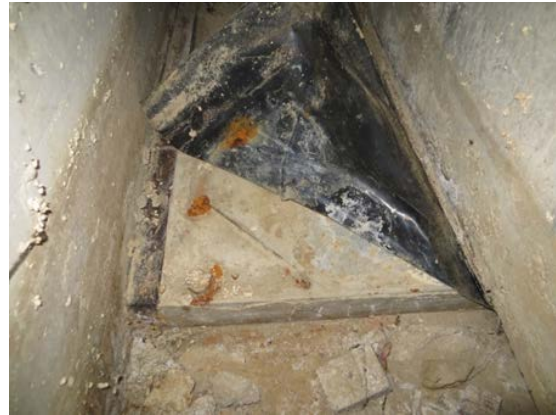
Figure 8. A view of a horizontal stainless steel plate with its protective plastic sheet folded back. When installed 20 years ago the stainless steel would have had a mirror finish. The coefficient of friction will be far greater than that assumed by the designers. (Chris Gannon)
