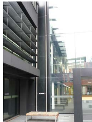
Figure 6. Rankin Brown Building, Wellington. The vertical black painted thin metal covering is part of the wall movement joint between the seismically-isolated building to the left and the fixed-base building to the right. Sacrificial steel elements and frangible interior linings will need replacement after a large earthquake.
