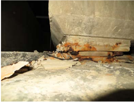
Figure 7. After 20 years exposure to moisture this pot sliding bearing is in urgent need of replacement. (Chris Gannon)
