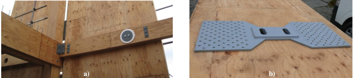
Figure 2. Connection of collector beams to walls. a) NMIT Building in Nelson with a large diameter pin (Devereux et al. 2011); b) Trimble Building in Christchurch with a steel-to-steel connection (Brown et al. 2012)
