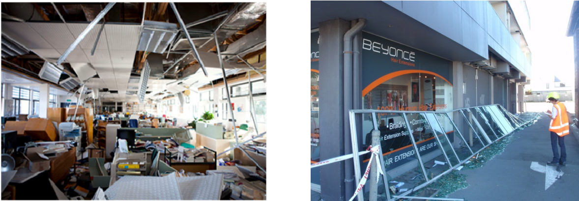
Figure 1. Widespread damage to a ceiling system (left), failure of a lightweight cladding system (right)
