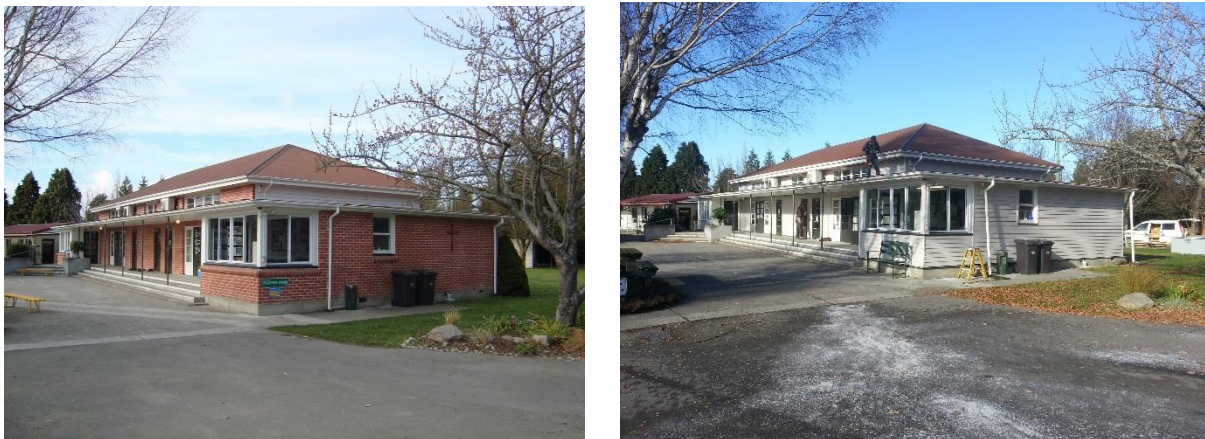
Figure 2. Before and after photo of a school showing replacement of brick veneer
