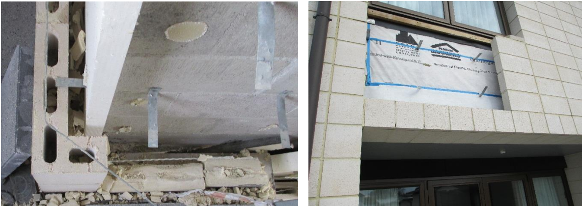
Figure 7. Photos of ineffective mortar tie joints
