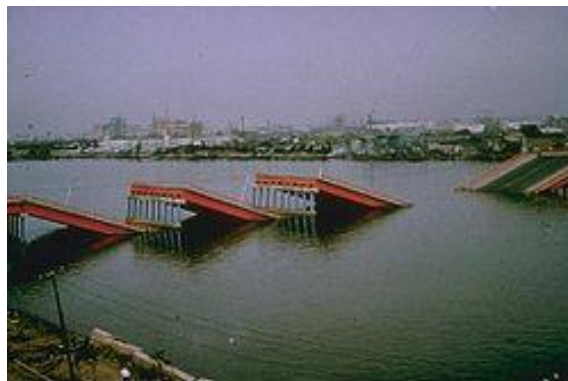
Figure 5. Collapse of Bridge in the Niigata Earthquake attributed to Liquefaction and Lateral Spreading
