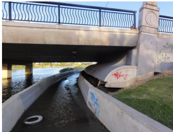
Figure 3. Damage to SH74 ANZAC Bridge in the Canterbury Earthquakes
