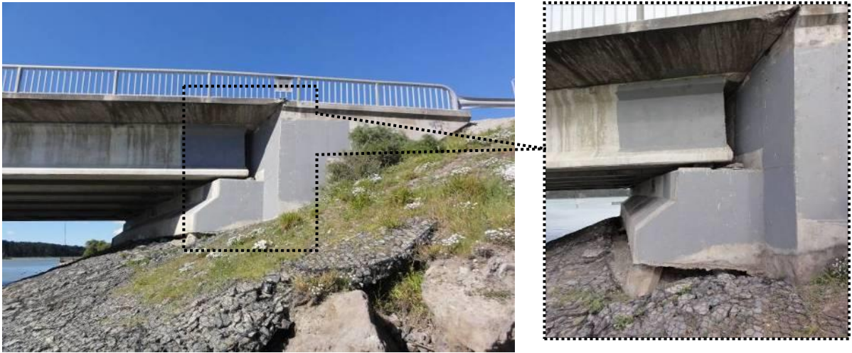
Figure 2. Damage to bridge abutment at South Brighton Bridge in the Darfield Earthquake of 4 th Sep 2010
