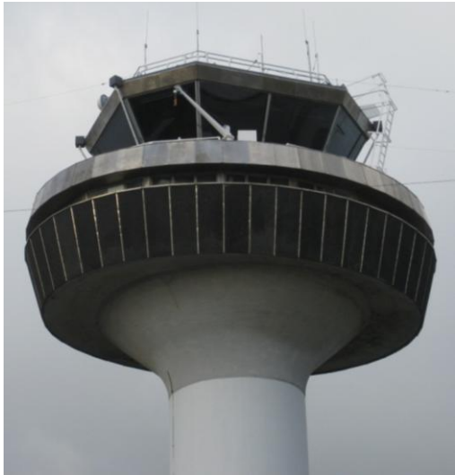
Figure 2: Close-up of service and cab levels
