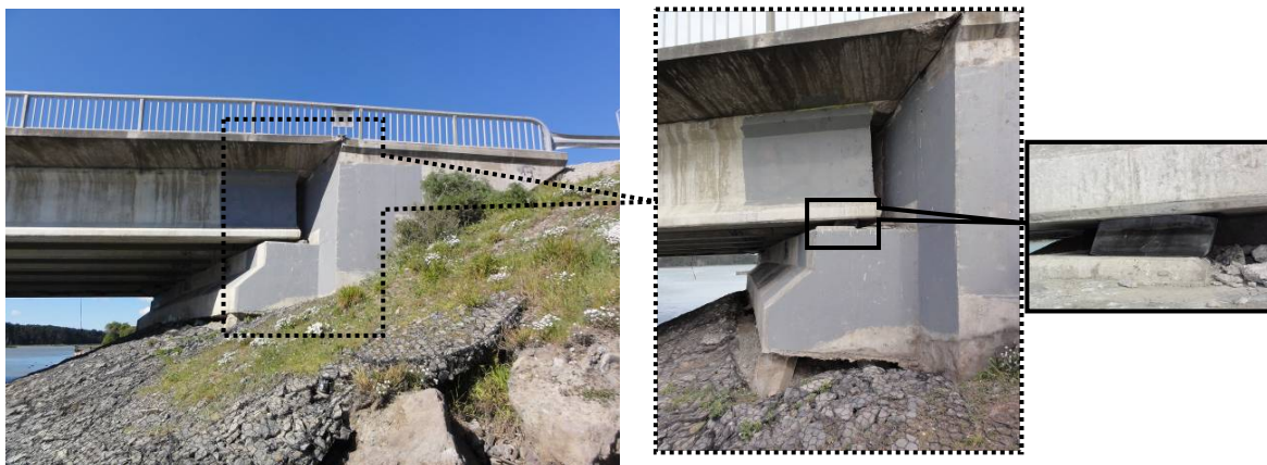
Figure 1. Damage to bridge abutment at South Brighton Bridge in 2010 Darfield Earthquake
