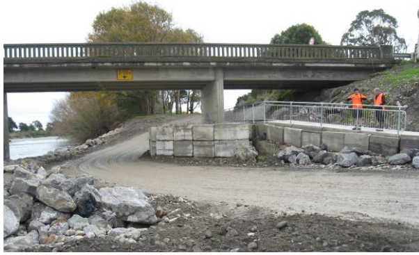
Figure 7. Rip rap and concrete blocks provide scour and earthquake protection at Otaki River Bridge
