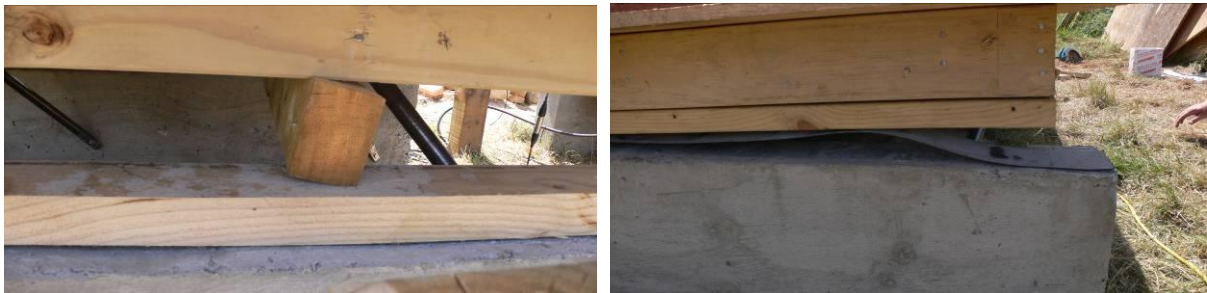
Figure 7. Left, failure of bearers in roll-over. Right twisting of other wall specimen
