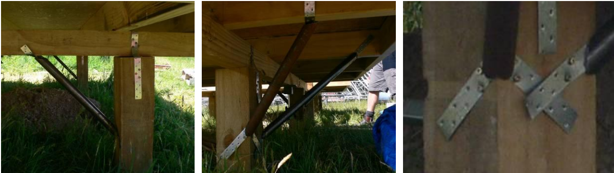
Figure 2. Steel pipe/nail plate connection, connected at 90° from pile to bearer (left) and at about 45° from pile to joists (centre) and close up of connection (right)
