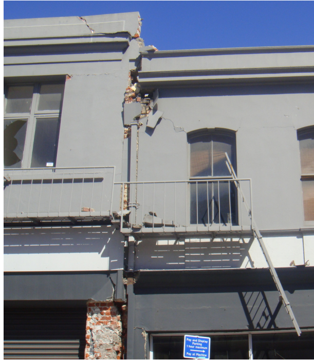
Figure 1. Pounding induced damage of buildings in Christchurch CBD
