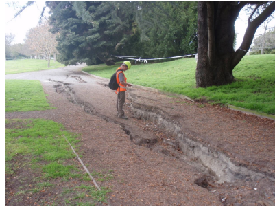
(b) Tracing crack with GPS
