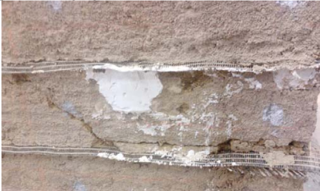
Figure 5.9 Crack running through geogrid layer on bottom right hand side of wall.
