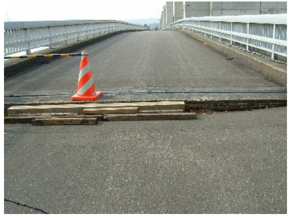
Figure 6. Approach road settlement at Koshino Bridge
