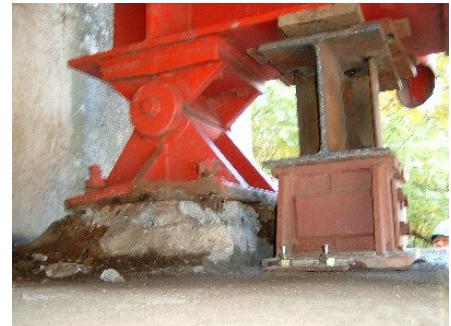
Figure 8. Temporary support at one of the damaged bearings, Miyanaka Bridge
