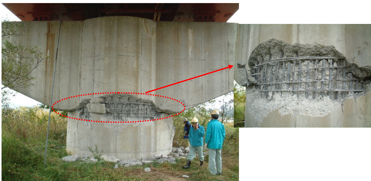
Figure 14. Damaged pier column, Ojiya Bridge (Photo courtesy of H. Nishida, PWRI)
