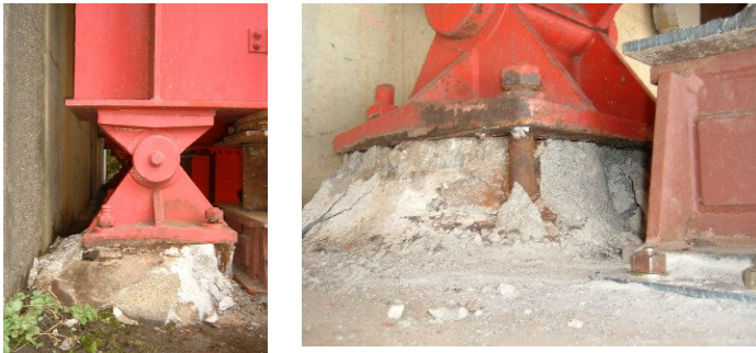
Figure 7. Damage to bearings of Miyanaka Bridge
