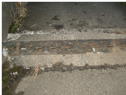
Figure 12. One of the damaged joints on Uonuma Bridge
