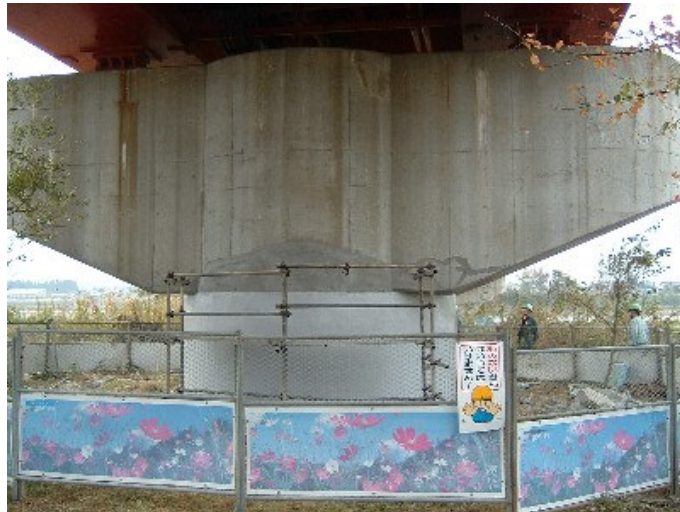
Figure 15. Column repaired with carbon FRP sheets, Ojiya Bridge (Photo courtesy of H. Nishida, PWRI)
