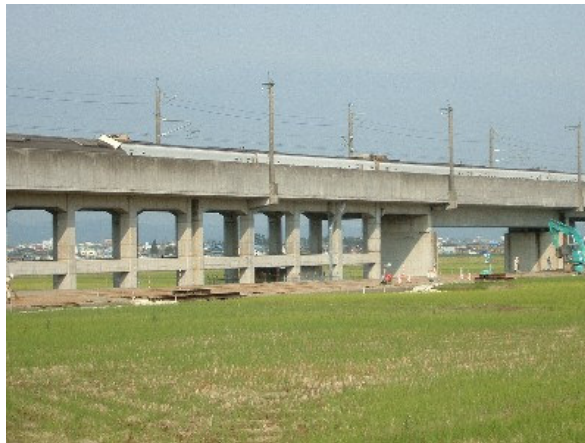
Figure 18. Katada Viaduct with derailed bullet train
