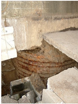
Figure 10. Pile pull-off, Yamabe Bridge
