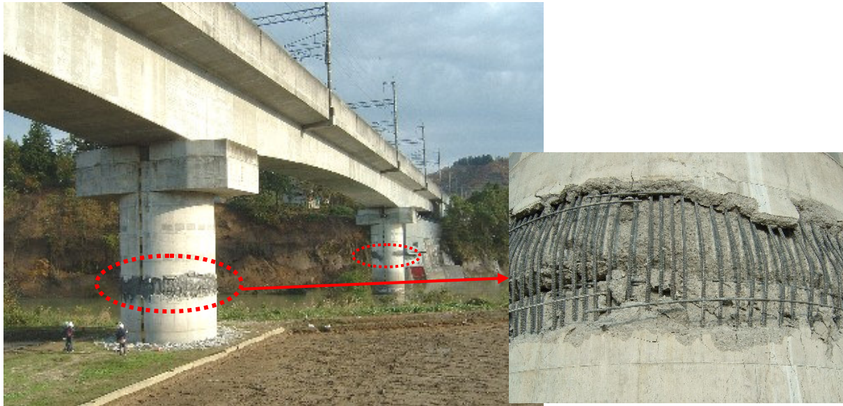
Figure 13. Flexural hinges developed at mid height of pier columns, Uonogawa Bullet Train Bridge
