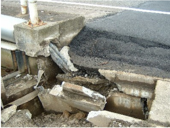
Figure 5. Approach road settlement at Hurumiya Bridge
