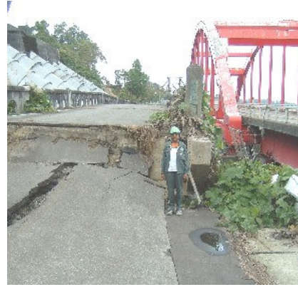
Figure 11. Soil slumping at Yamabe bridge site
