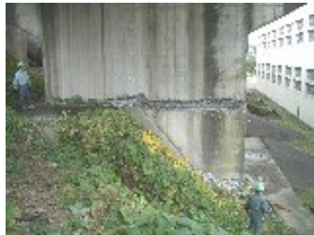
Figure 16. Damaged wall pier, Yamabe Bridge
